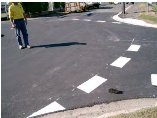
Installed ready for use
